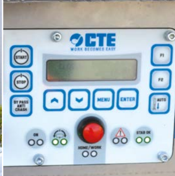
DIAGNOSTIC TOOL INTEGRATED IN THE CONTROL PANEL
